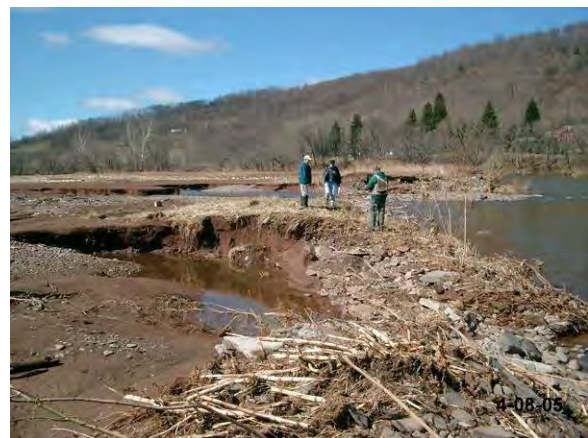
Figure 3.11 Berm that was breached in 2005 storm event
