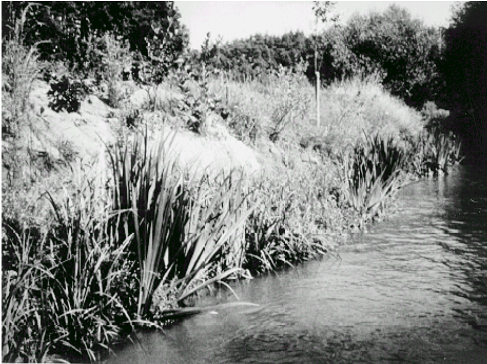
Figure 5.23b. Coir roll planted with vegetation (photo courtesy of Bestmann GmbH, Wedel, Germany)
