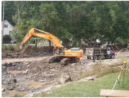
Above: An excavator removing excess gravel from the Stony Clove in the days following the flood.
